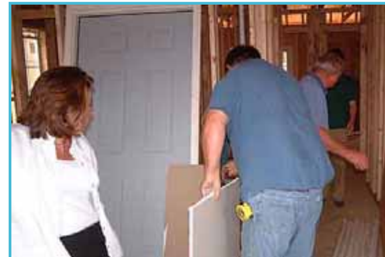
Ashley Bowie (left), housing transition manager, pauses to let CRDC employees Allen Orr, Ronald Martin and John Griffith pass during a tour of the new apartment complex under construction by the agency in Jonesboro. The CRDC crew was installing heating and cooling ducts.
